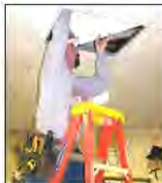
Workers install new wiring at YHS. Multimedia projectors will be hung in each classroom teacher's room.
